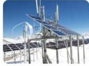
Mountain communication base station
