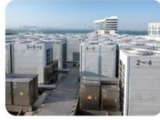
communication base station energy storage
